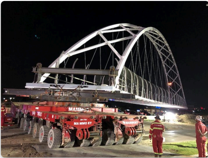
Mammoet teams moved the Northaven Trail Bridge into place over of a weekend.
